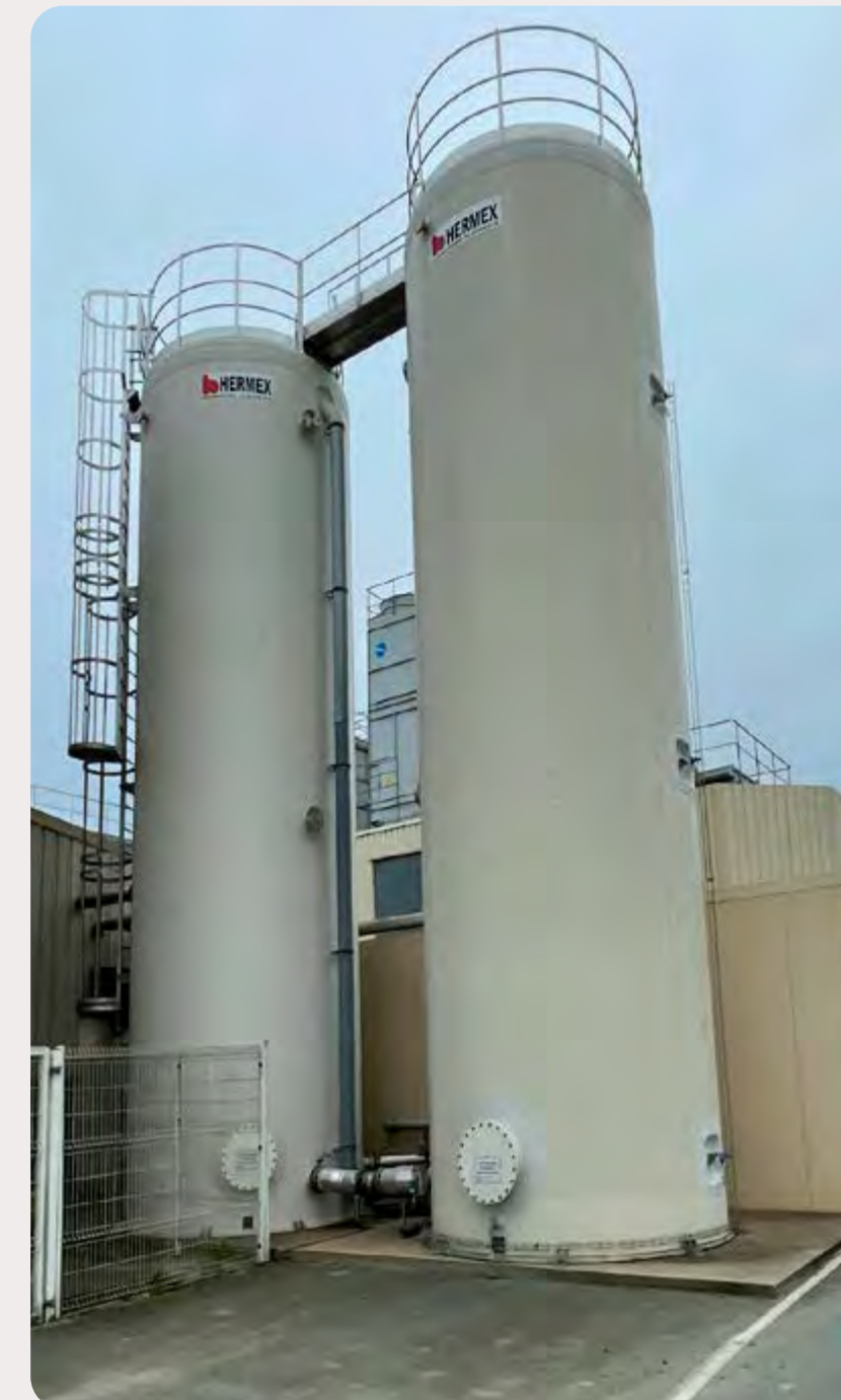
Two water tanks of 75m 3 at our site in Gourin, to store the site's hot water. The water is heated with residual heat
